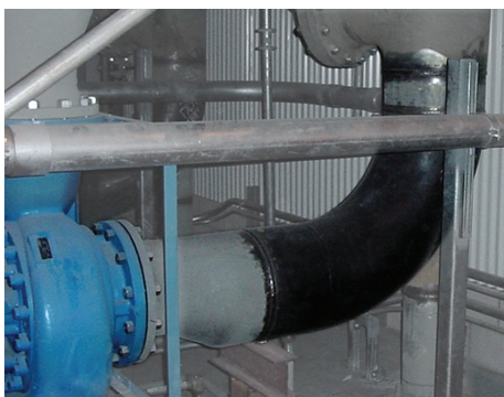
Vortab VEL installation at pump inlet
