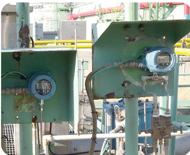
Natural Gas Monitoring
