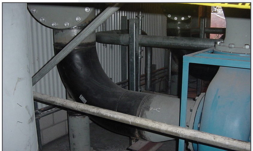
Figure 4: Electric Power Plant Elbow and Pump
