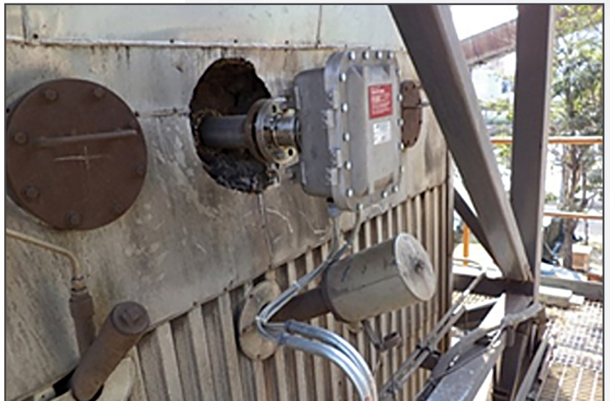
Figure 3B, bottom: Extreme example of very large diameter pipe, high temperature insulation, dusty, outdoor, above ground installation point, and in Div.1/Zone 1 type Ex location that were made clear at the beginning to ensure first time right success.
