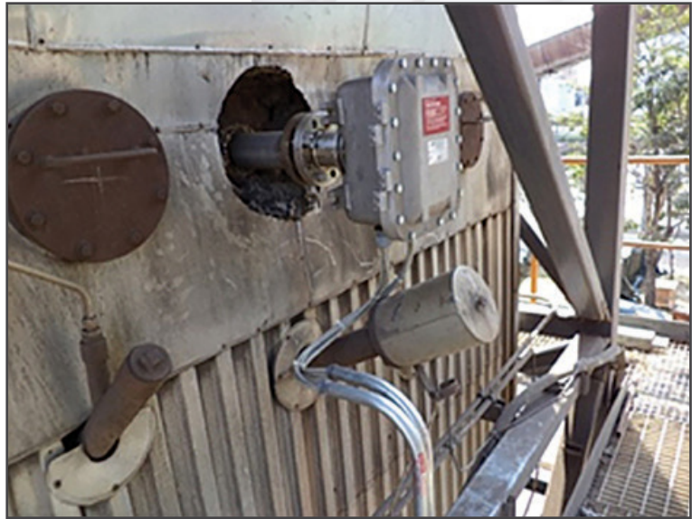
Flue gas monitoring at a cement plant
