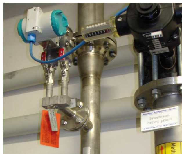
Deployment of deltaflow for biogas flow metering.
